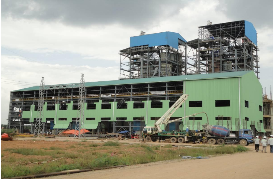
Bangunan Steam turbine generator, boiler 1 dan boiler 2
